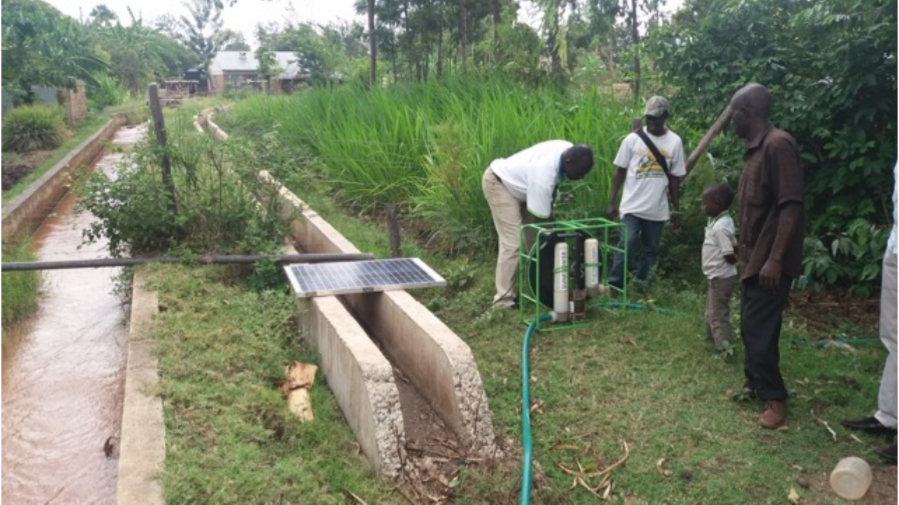
Solar pump at the demonstration farm near Kendu Bay.
